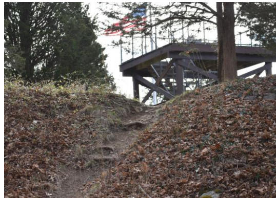
Photo: Erosion on the steep slopes from pedestrians and bikes could be the beginning of irreparable damage to the fort slope.
