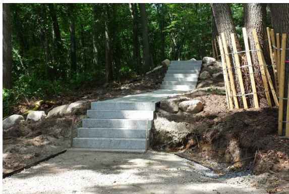
Granite step access under construction at historic Greene Cemetery, Warwick RI Designed by Bradford Associates
